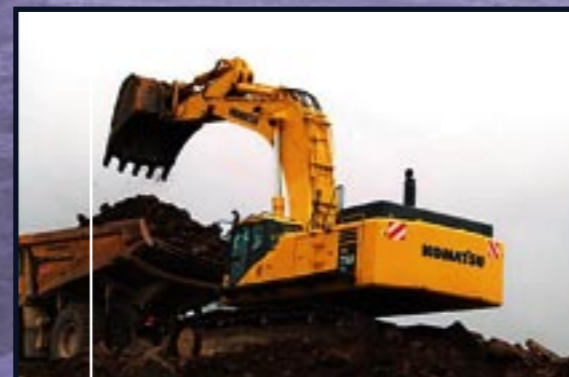
An 80-tonne Komatsu PC750-7 excavator is also in operation at this site.
