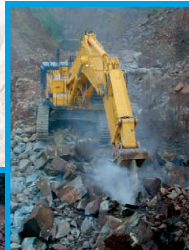
The ripper tooth – interchangeable with the bucket – breaks up the stone. Blasting would damage the stone.
