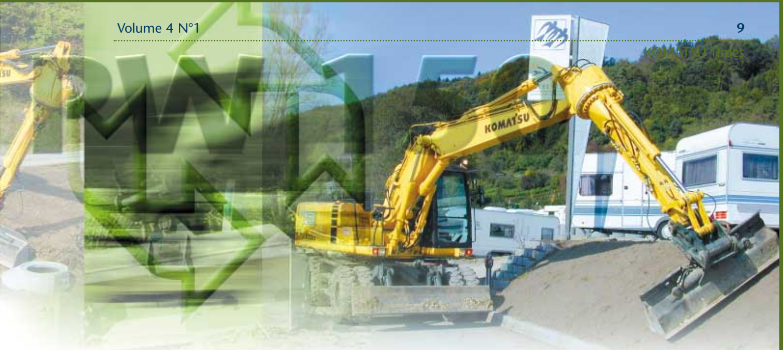
Complex slopes finished in one operation thanks to the rotating arm and swing bucket.
