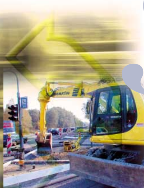
The mobile excavator distributes concrete on a traffic island. The rotating arm follows the complex contour of the traffic island, and the operator doesn't have to move the machine.
