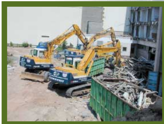
Komatsu crawler excavators, wheeled excavator and a wheel loader sorted material and loaded lorries
